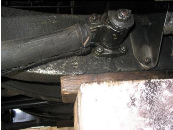
Fig 1 Supporting the axle directly under the chassis. A good firm and well located support just forward of the front end spring shackle
