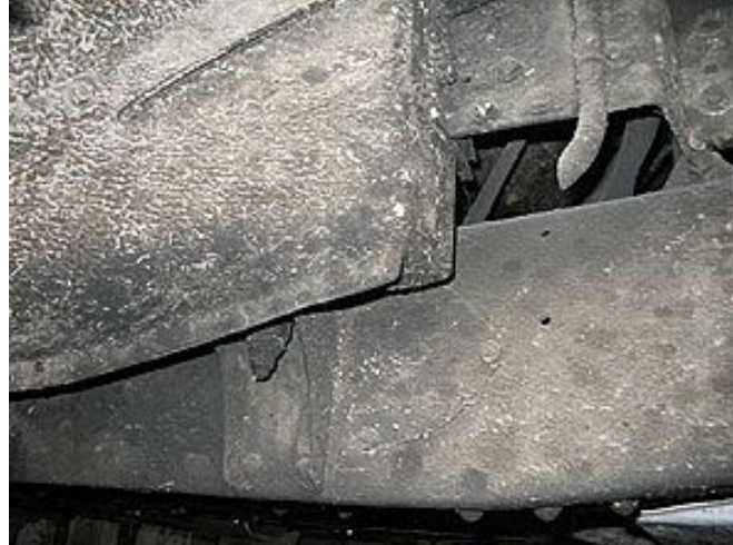
Front end of sill under front wheel arch should be checked thoroughly for rust.
