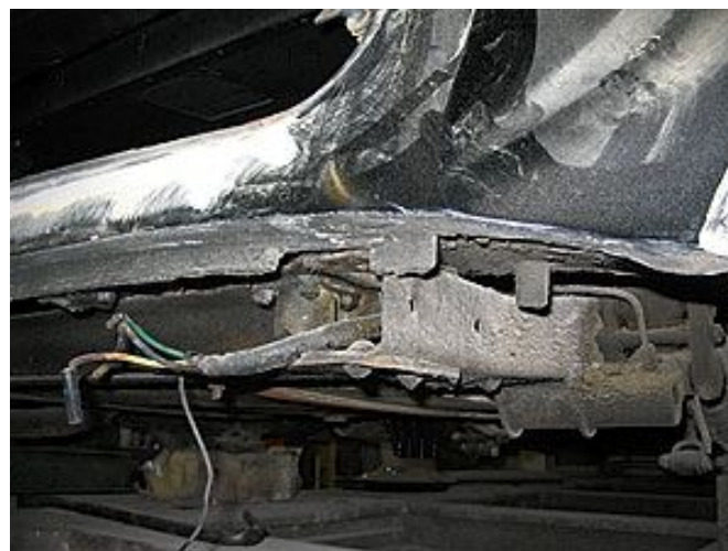
Body sitting on chassis at rear because body mount has collapsed
